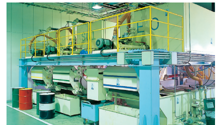
Cutting liquid recycling system
