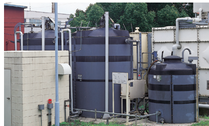
Wastewater treatment system
